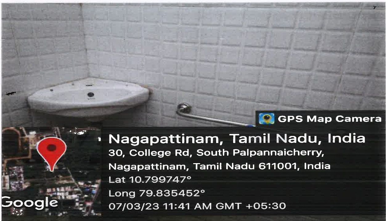
Disabled free washroom
