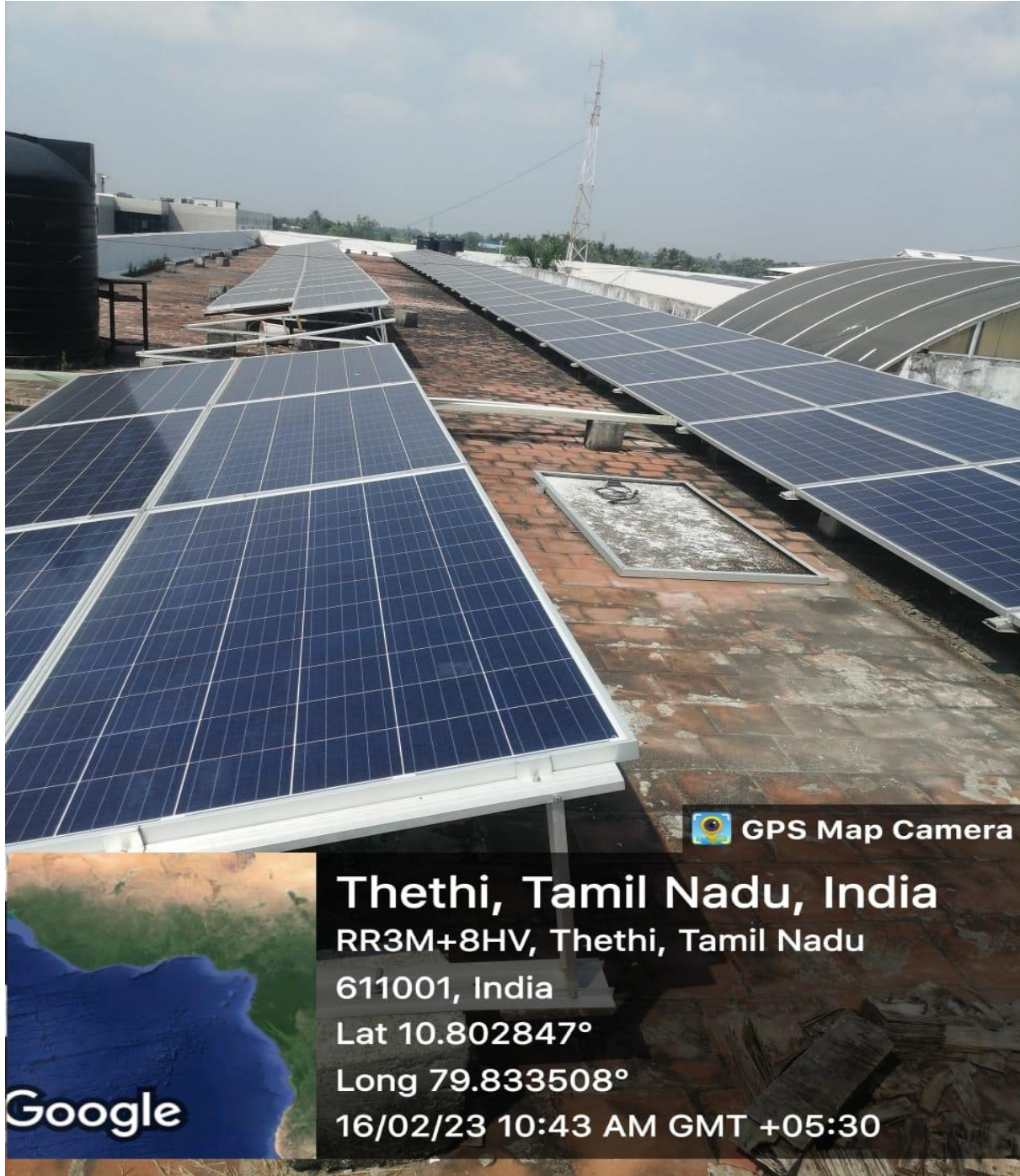
Solar PV plant (GG Block)
