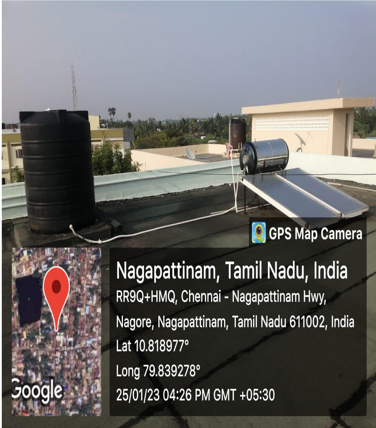
Solar Water Heater
