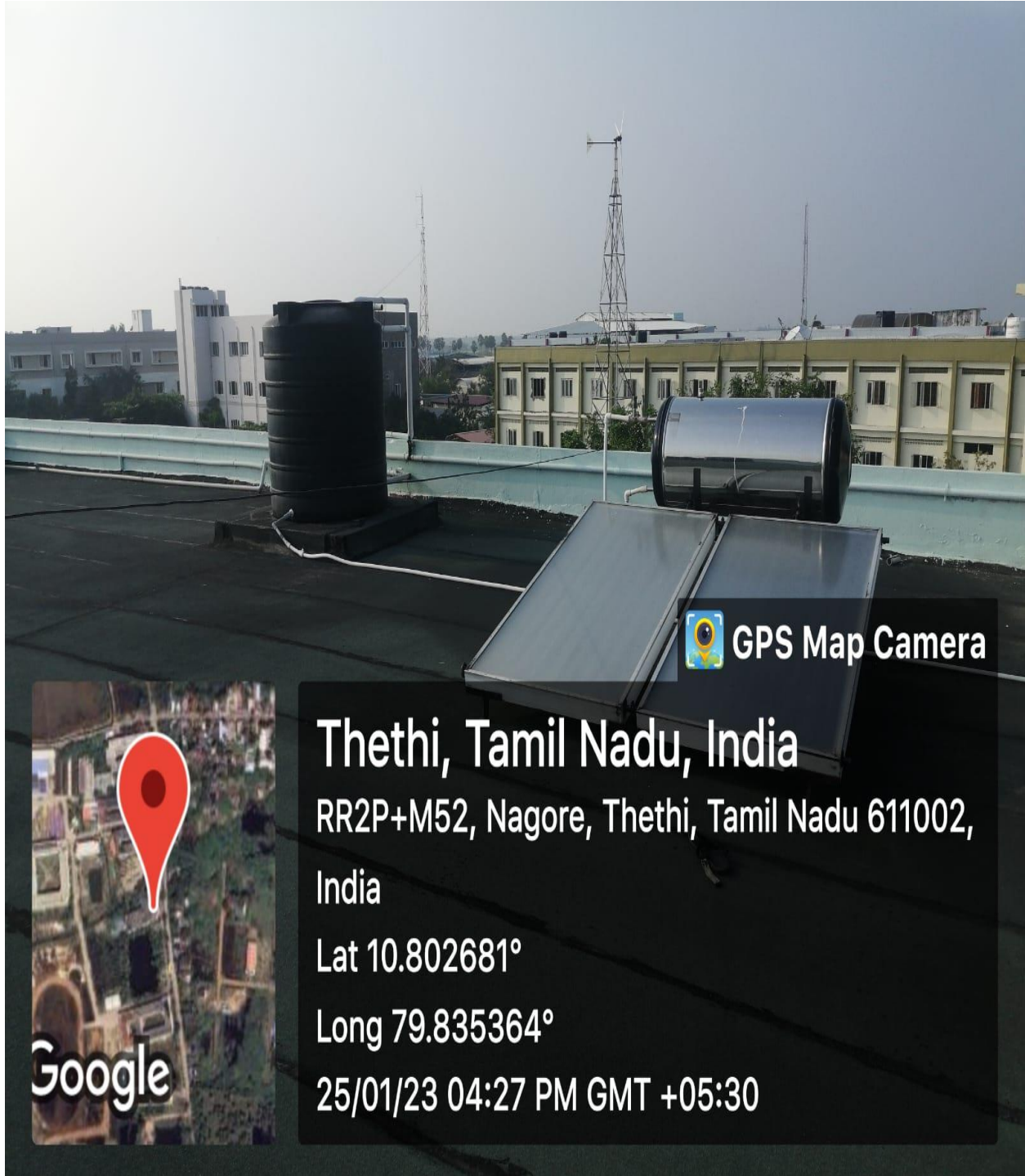
Solar Water Heater
