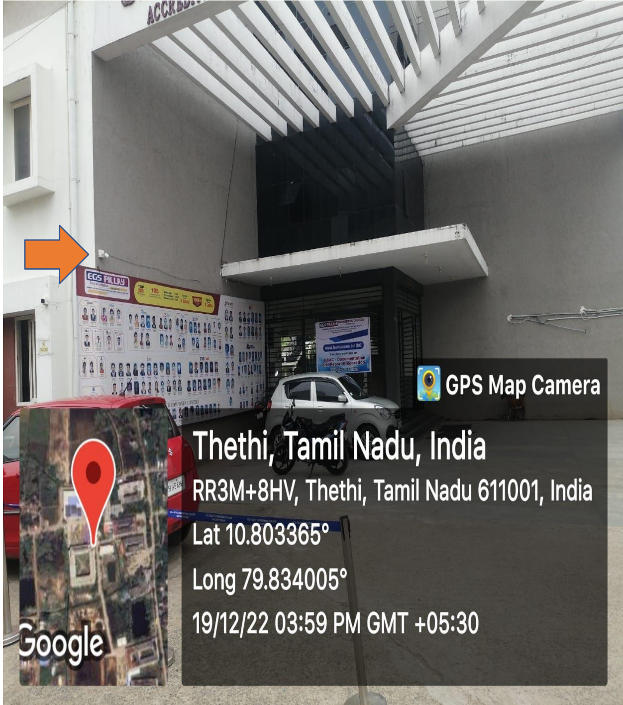
Outdoor CCTV Camera (SJ Block)
